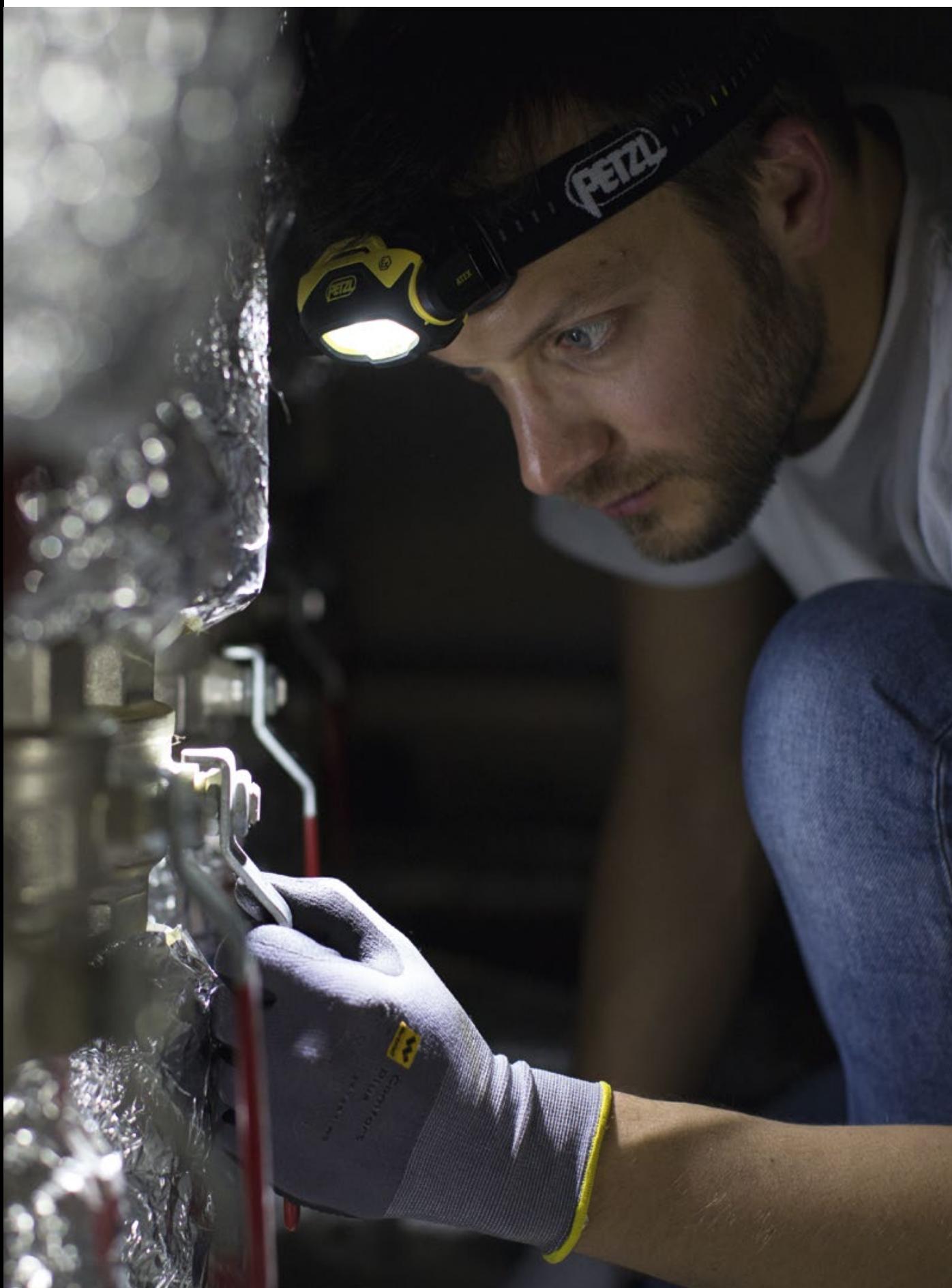
Boiler room inspection and maintenance © Petzl - Lafouche
